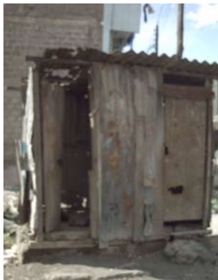
a dilapidated school latrine
